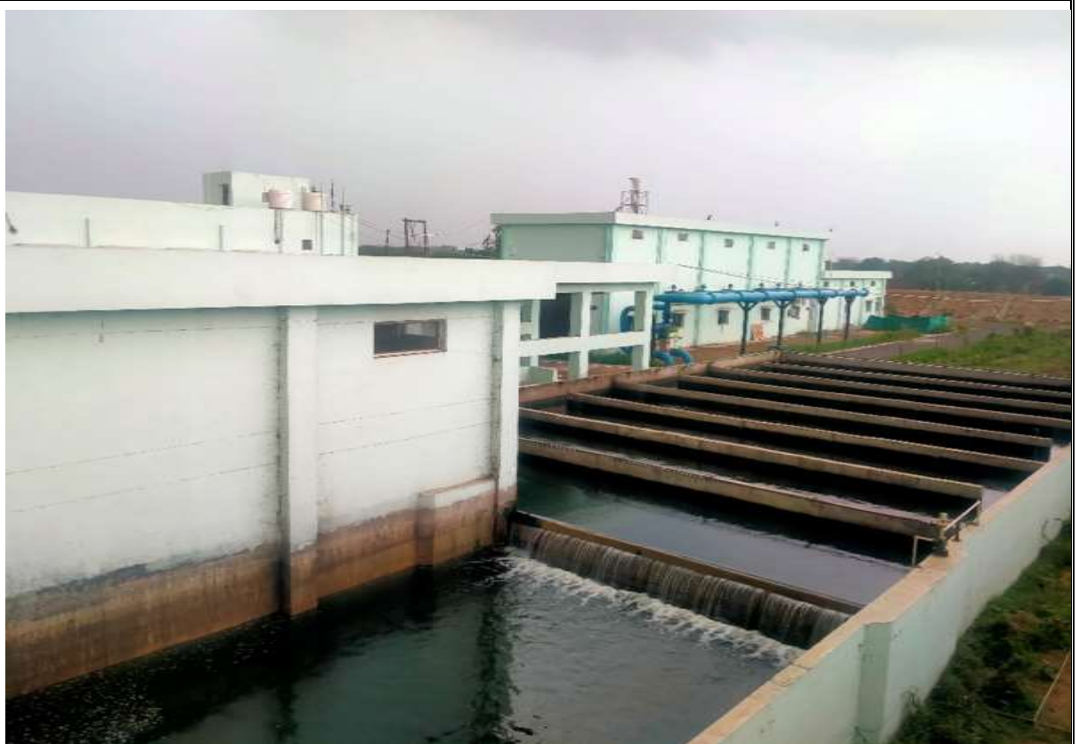
Quality of Treated Effluent at Treated Water Collection Tank ,STP
