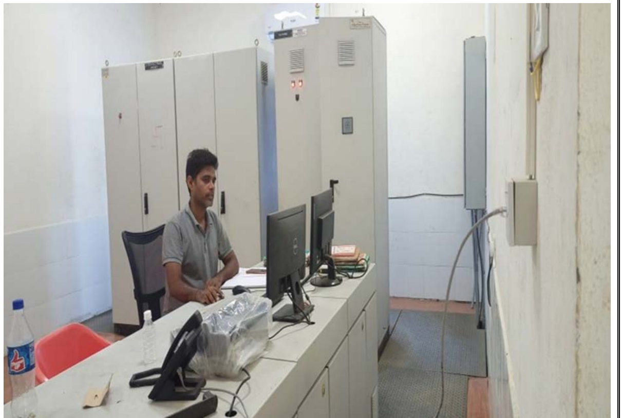
PLC & SCADA Room @ STP
