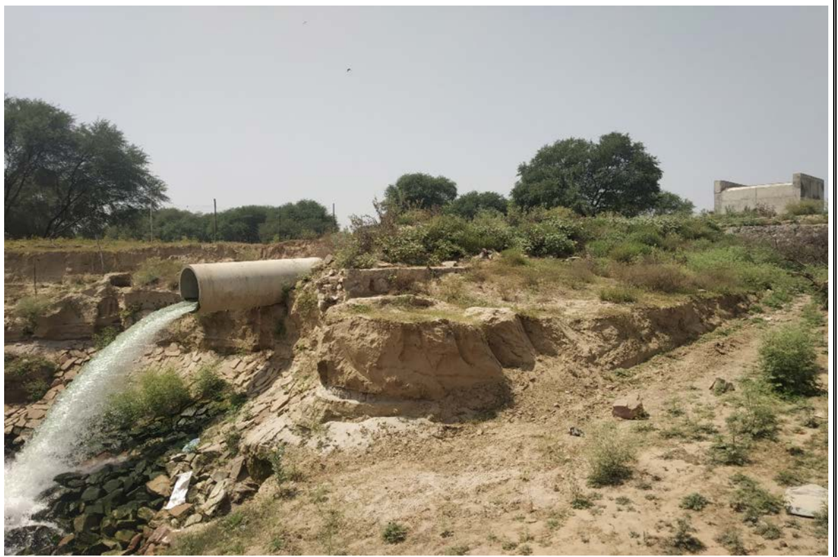
Treated effluent disposal
