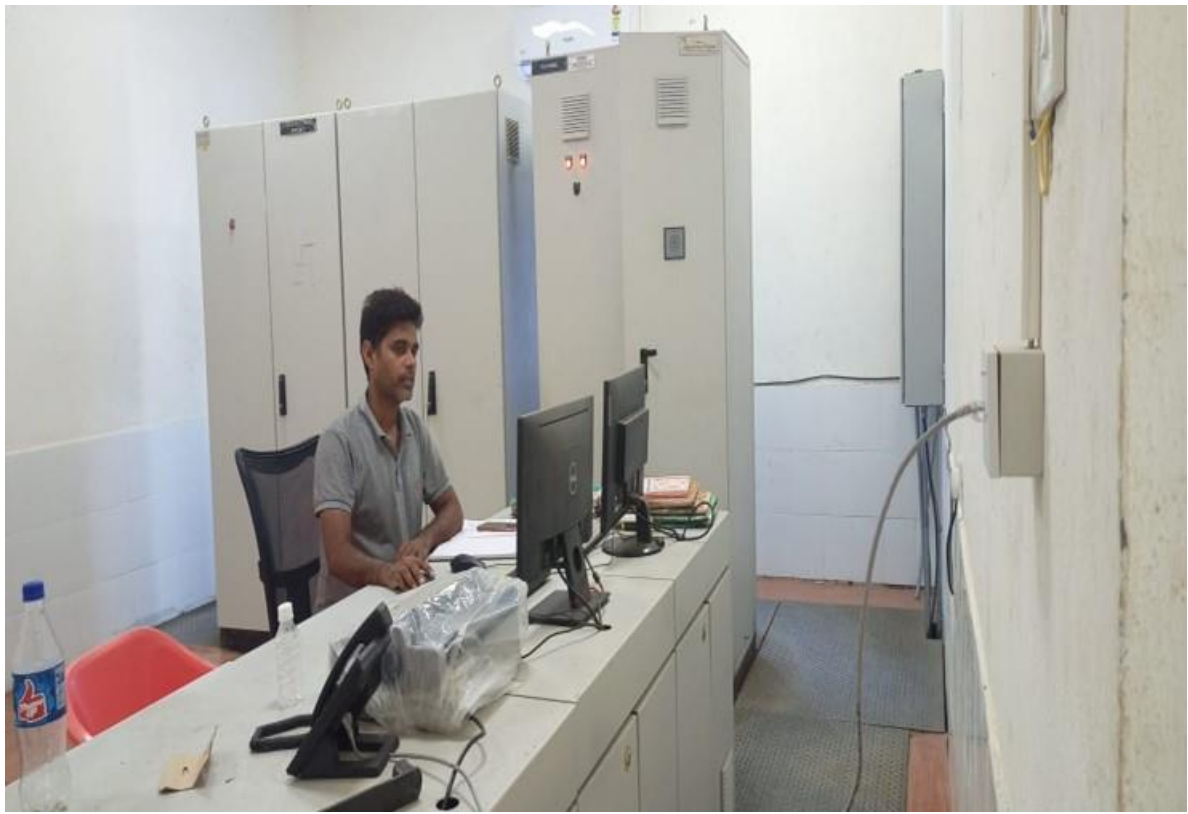
PLC & SCADA Room @ STP
