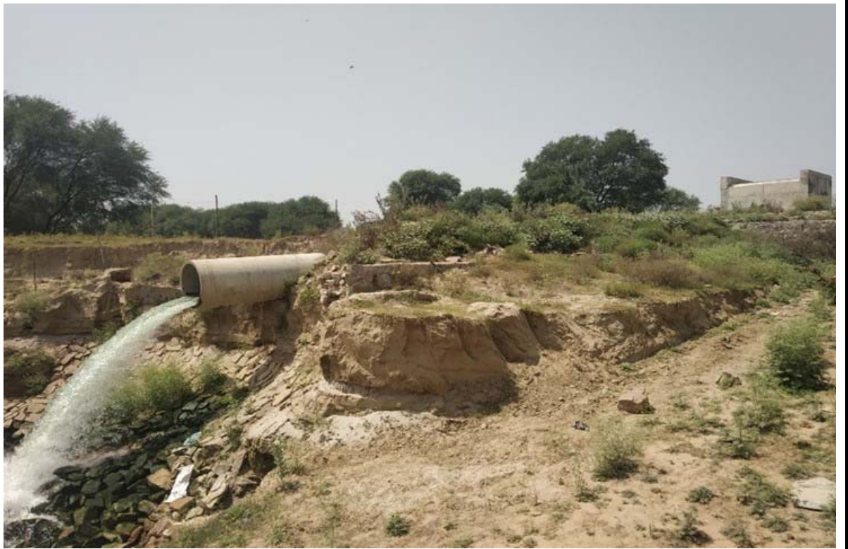
Treated effluent disposal
