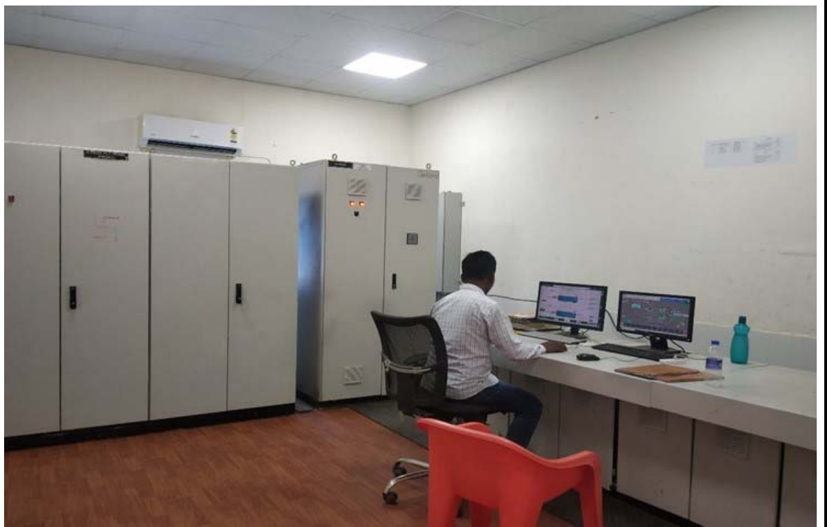
PLC & SCADA Room @ STP
