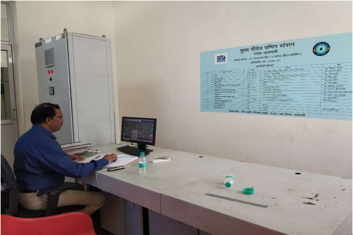
PLC & SCADA Room @ MPS
