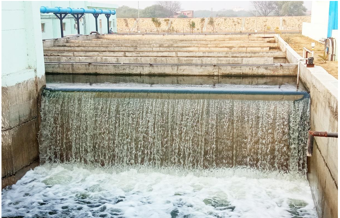
Quality of Treated Effluent at Treated Water Collection Tank ,STP
