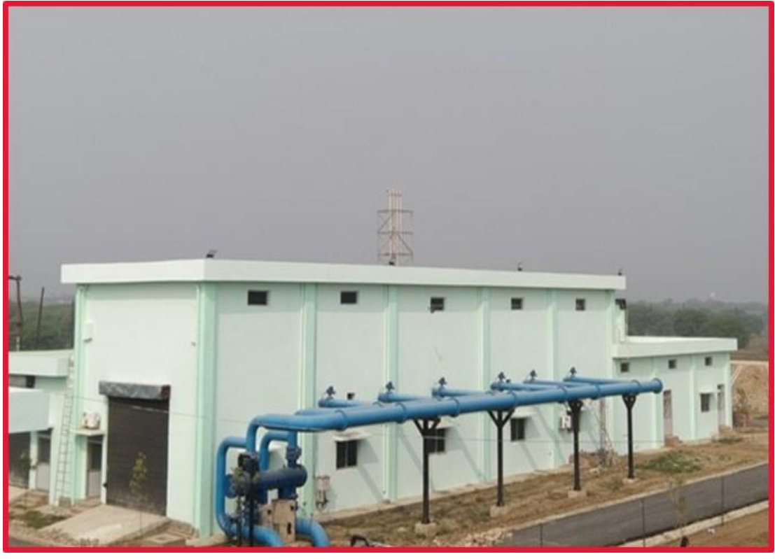
Airblower, HT, PMCC room & DG Shed area-Side View
