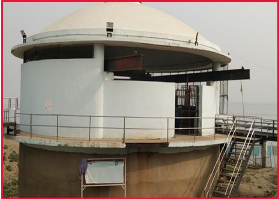
MPS Wet Well and Dry Well,
