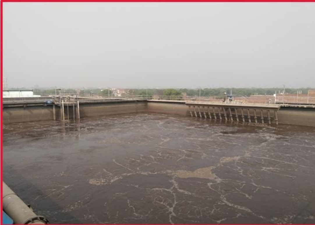
Aeration @ SBR Basin
