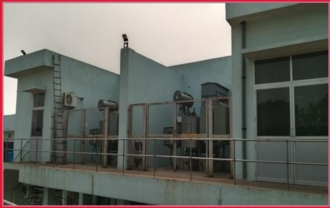
Transformer Yard, MPS
