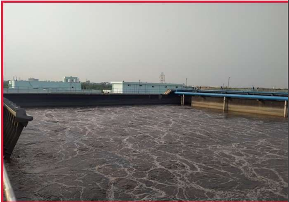
Aeration @ SBR Basin
