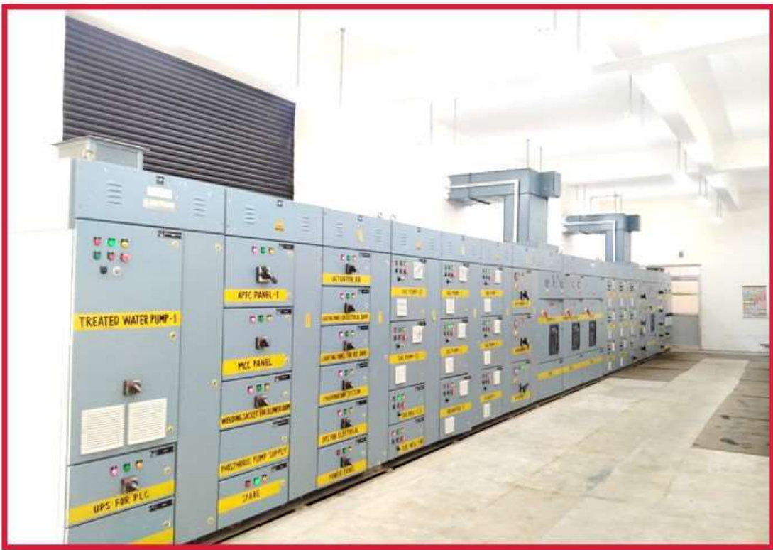
PMCC Panel @ STP
