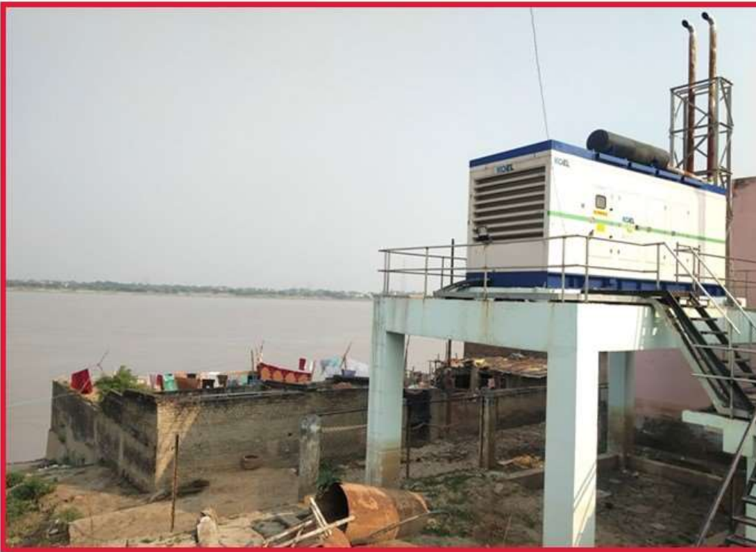
625 KVA DG Set @ MPS
