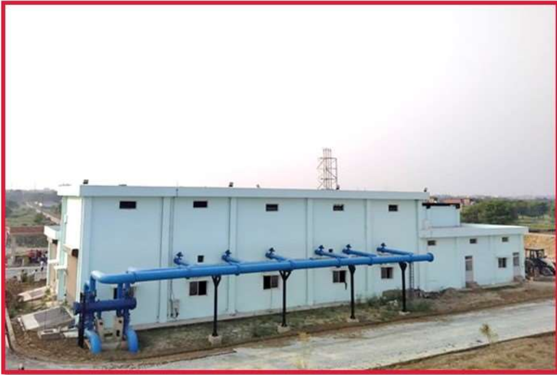
Airblower, HT, PMCC room & DG Shed area-Side View
