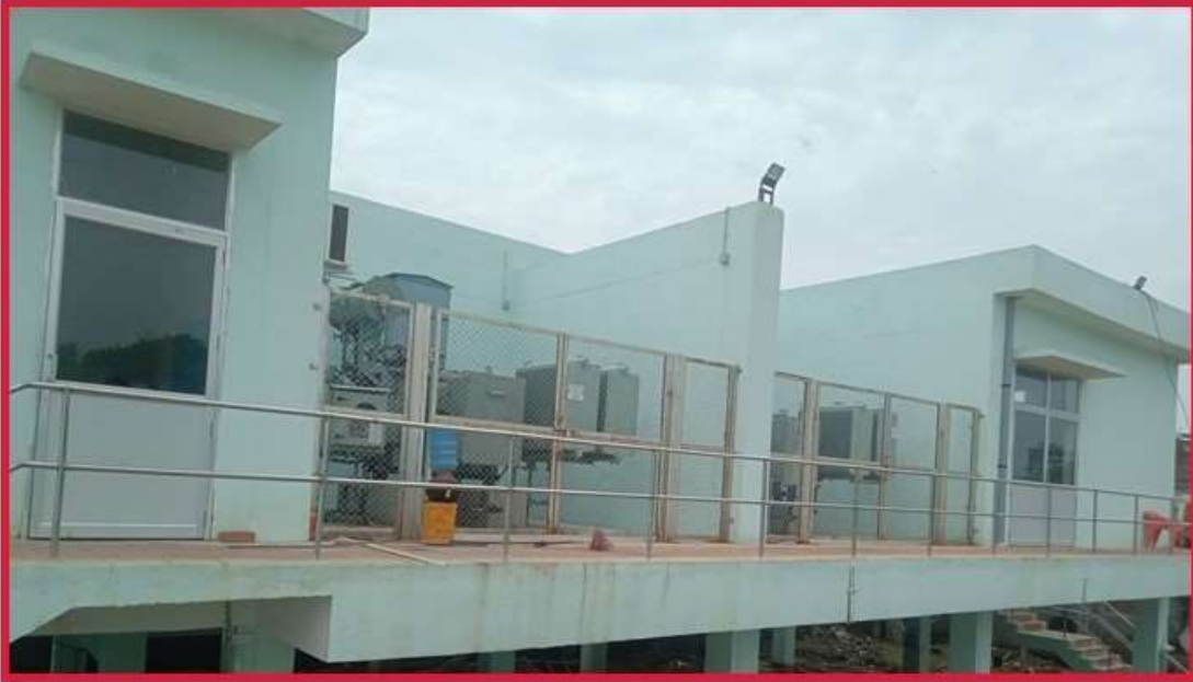
Transformer Area @ MPS
