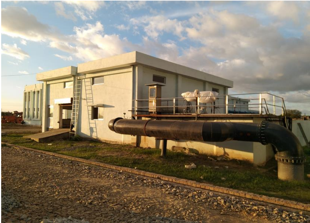
Airblower, HT room, MCC, PMCC & DG Shed
