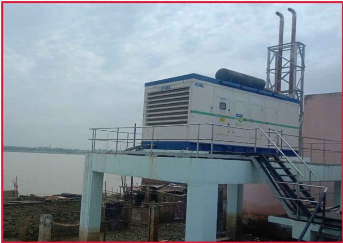
625 KVA DG Set @ MPS
