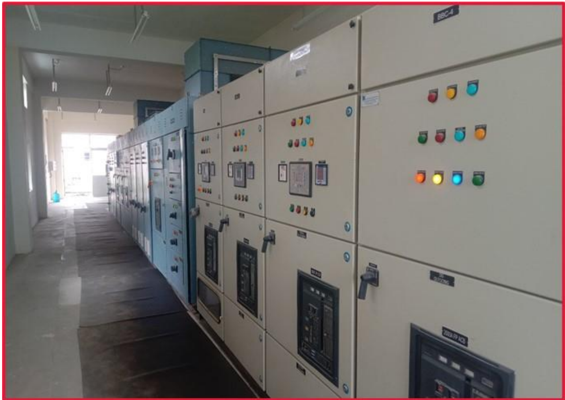
PMCC Panel Room @ MPS
