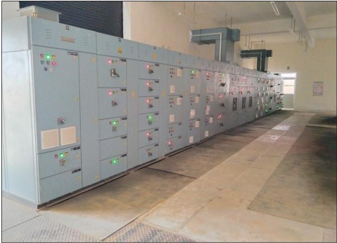
PMCC Panel @ STP
