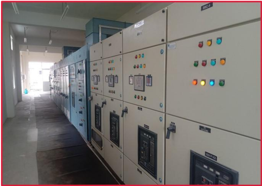
PMCC Panel Room @ MPS
