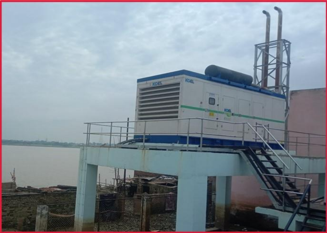
625 KVA DG Set @ MPS
