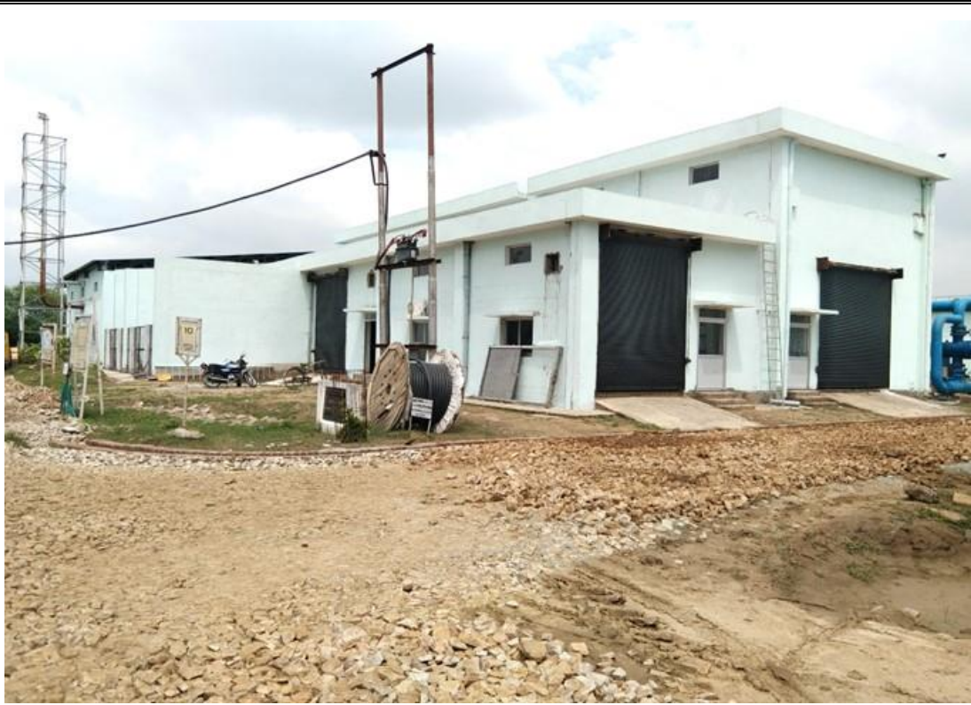
Airblower, HT room, MCC, PMCC & DG Shed
