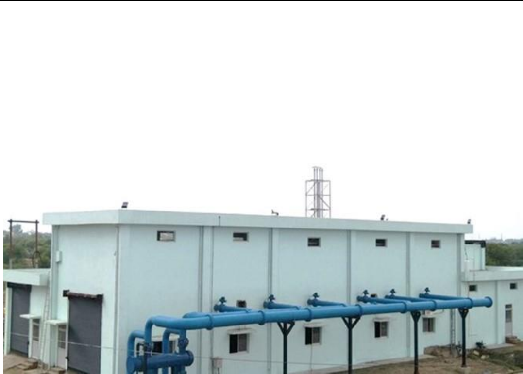
Airblower, HT room, MCC, PMCC & DG Shed
