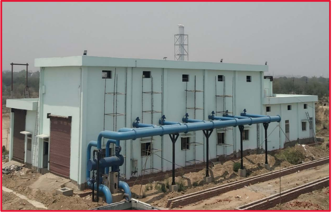
Airblower, HT room, MCC, PMCC & DG Shed
