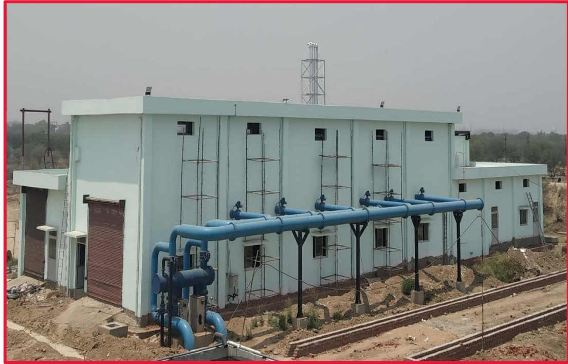
Airblower, HT room, MCC, PMCC & DG Shed
