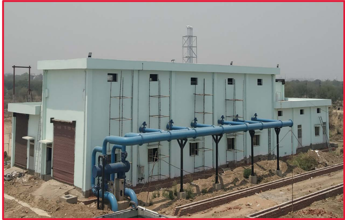
Airblower, HT room, MCC, PMCC & DG Shed
