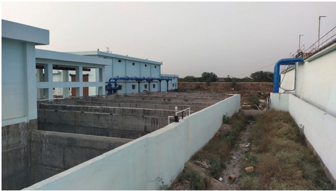
Chlorine Injector Pipe Line and Pump
