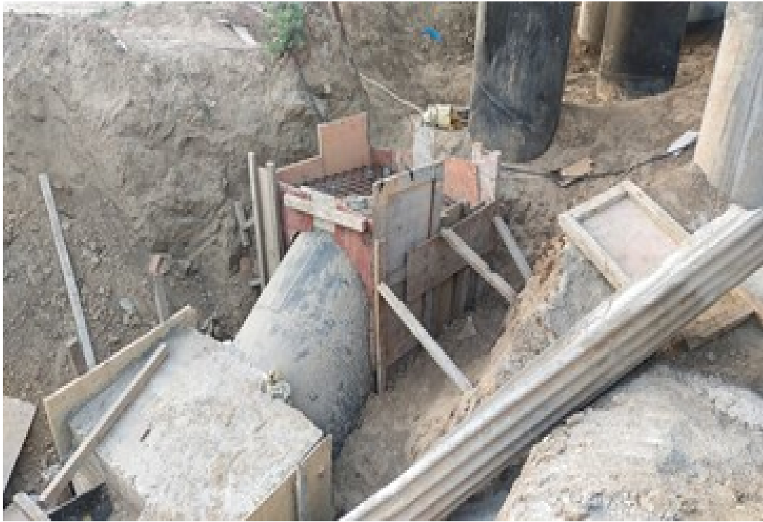
Thrust Block @ Treated Effluent Line
