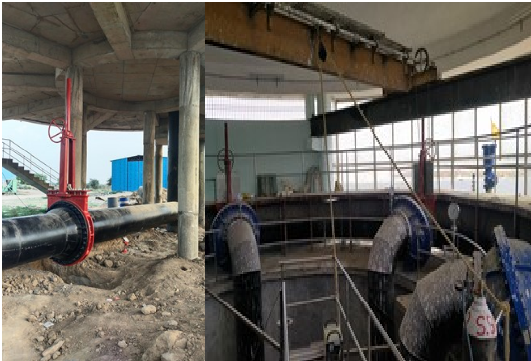
Erection KGV @ Bypass Line at STP & Fixing of pressure gauge on Discharge Line@Dry well, MPS
