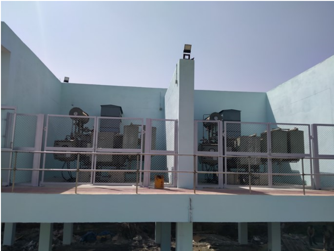
Fencing Gate for Transformer Yard - MPS
