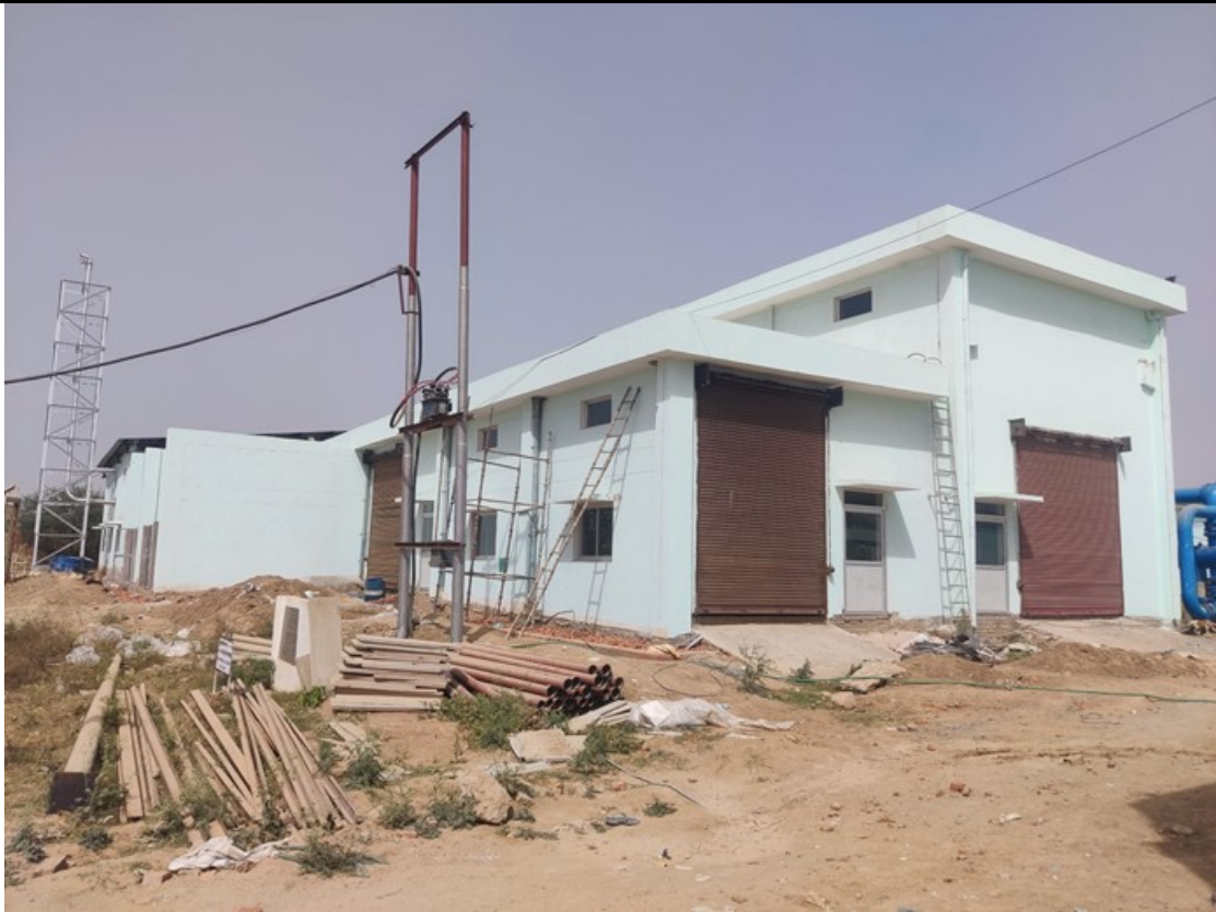
Airblower, HT room, MCC, PMCC & DG Shed
