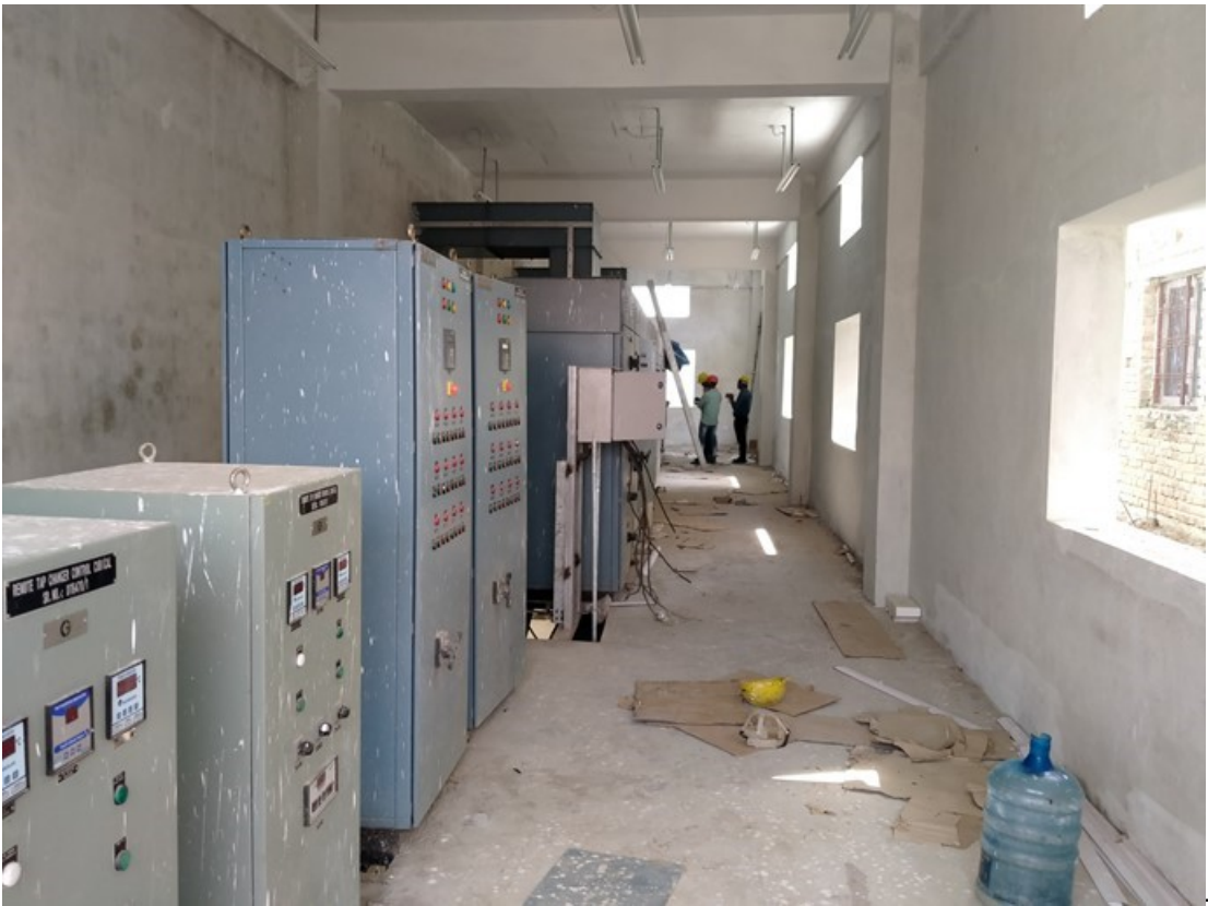
Panel room @ Electrical Control Room, MPS
