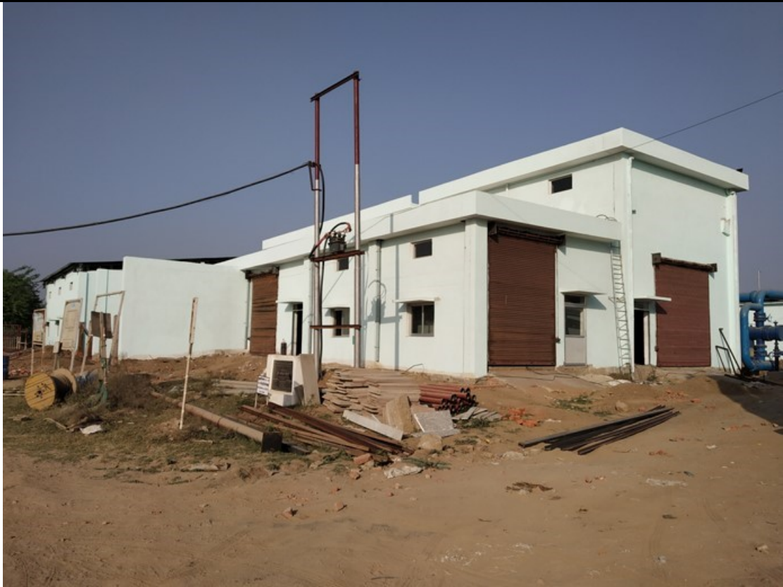
Airblower, HT room, MCC, PMCC & DG Shed
