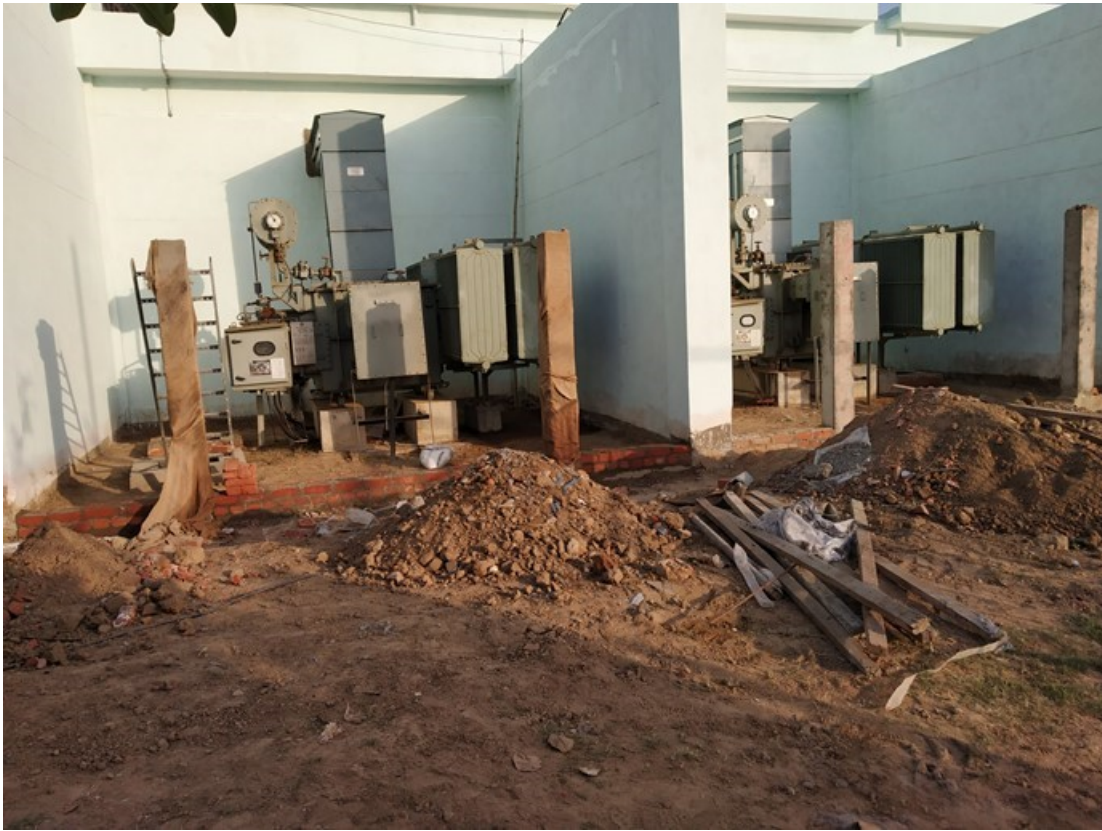
Transformer area at STP
