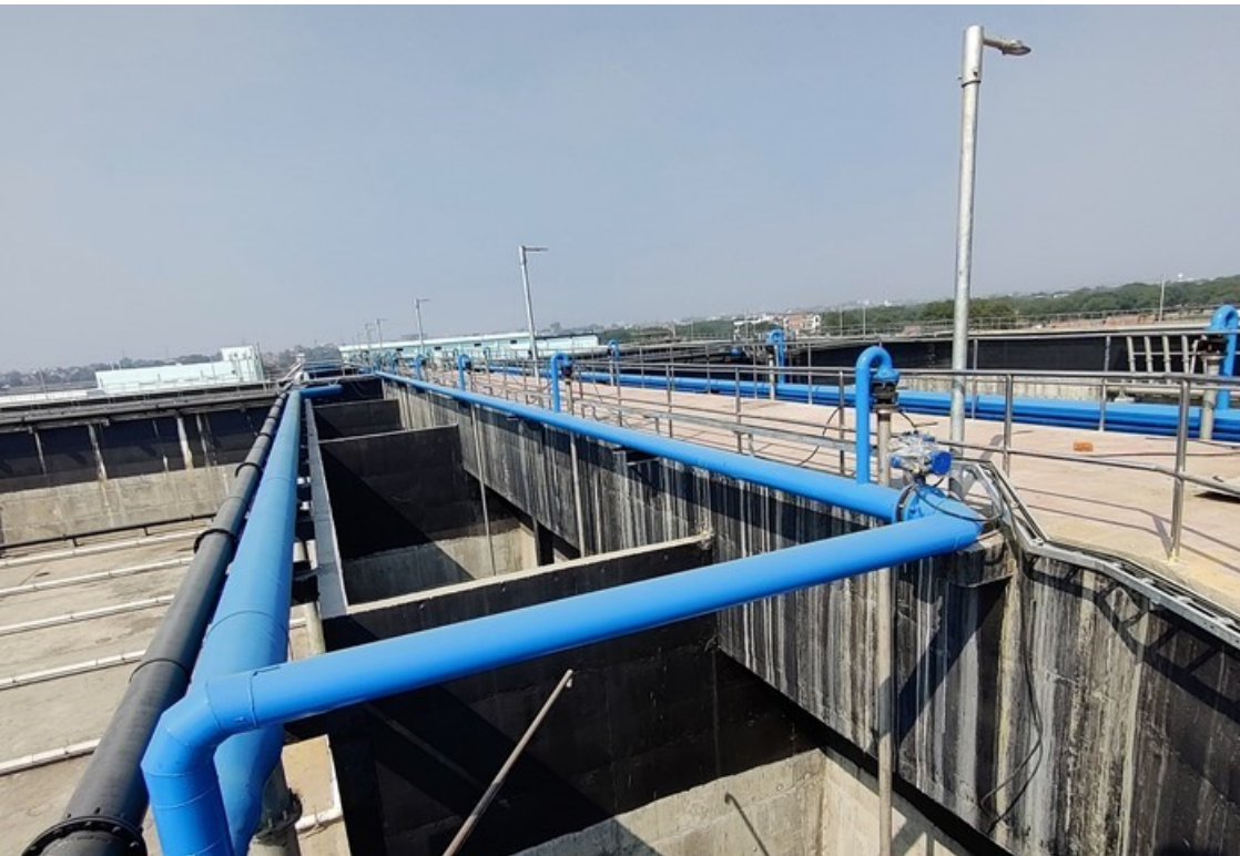
Airline Piping in Selector Zone@SBR
