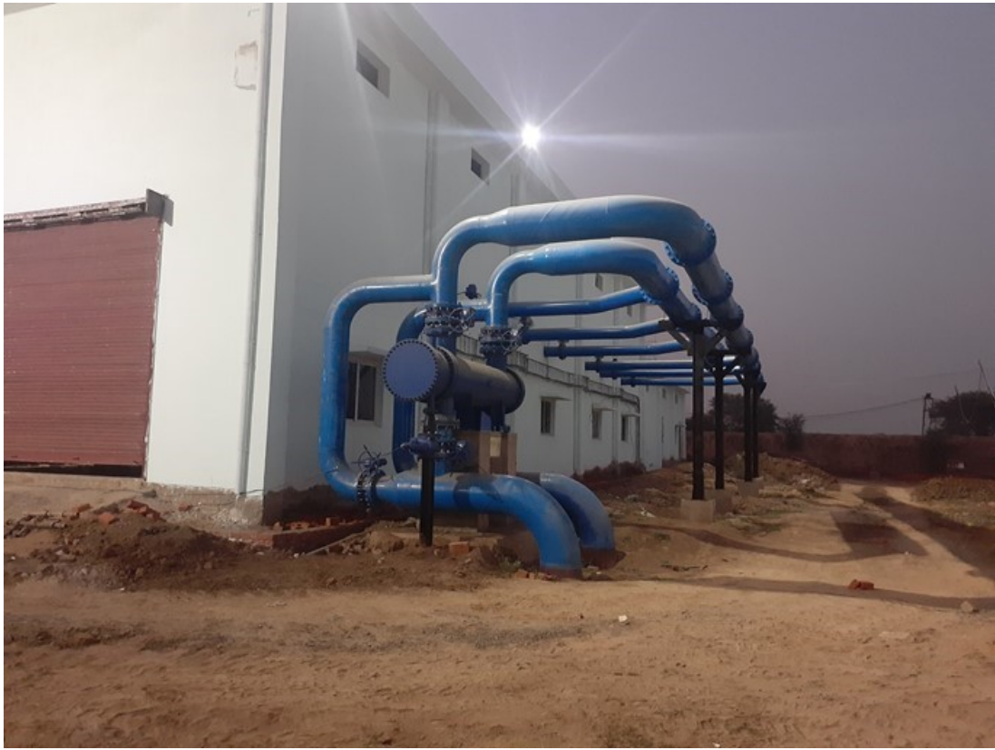
Heat Exchanger with Piping
