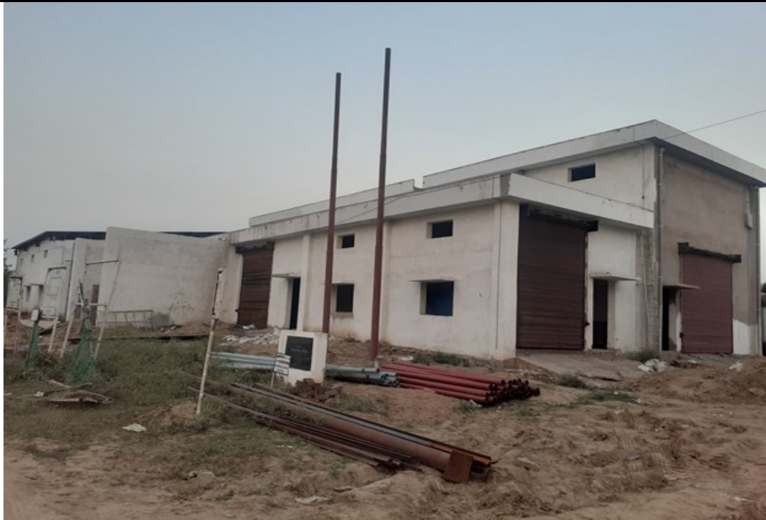
Airblower, HT room, MCC, PMCC & DG Shed
