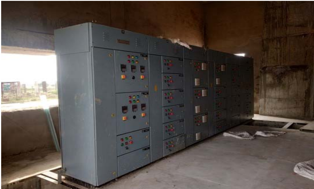
MCC Room – BFP building
