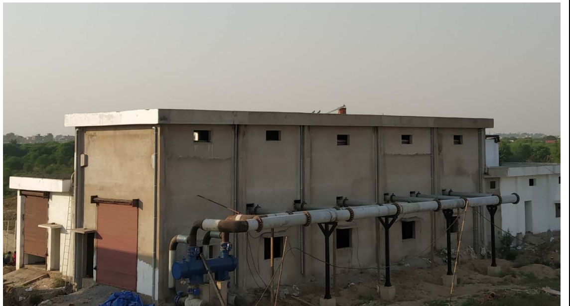
Airblower, HT room, MCC, PMCC & DG Shed
