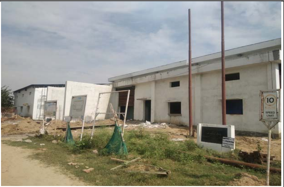
Airblower, HT room, MCC, PMCC & DG Shed
