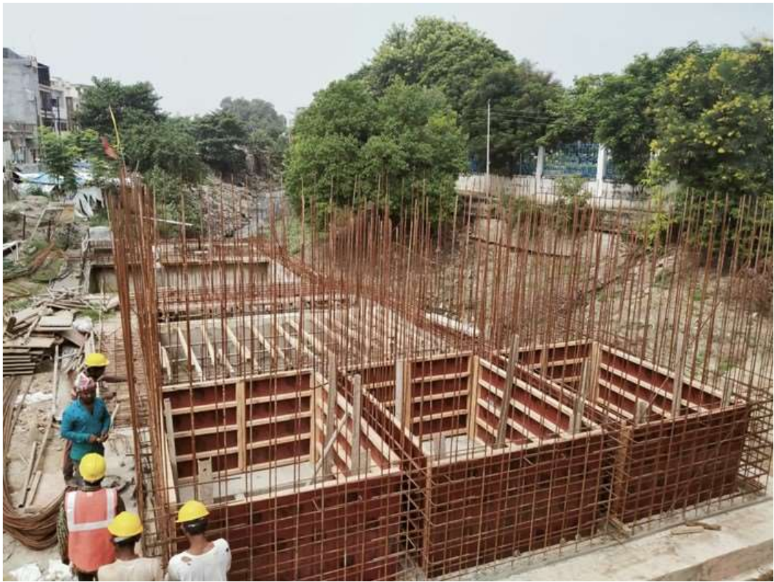
Receiving Chamber at MPS
