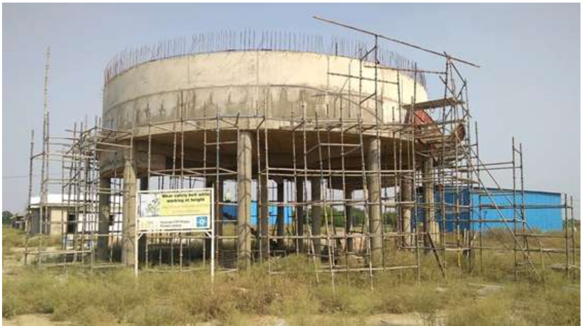
Overhead treated water tank
