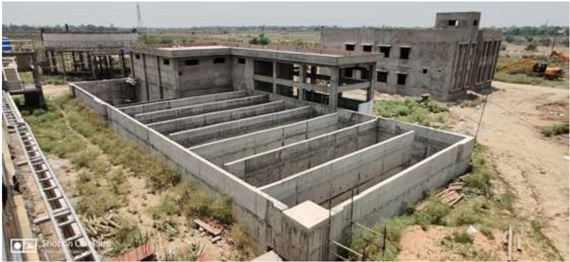
Chlorination contact tank
