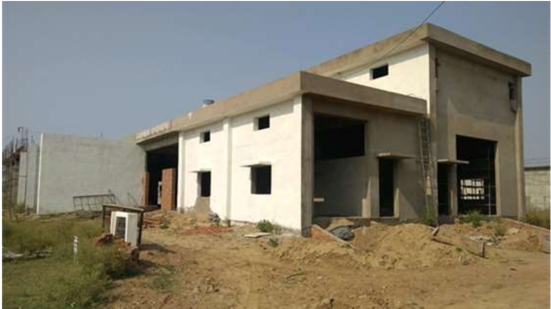
Air blower, PMCC, SCADA & HT room
