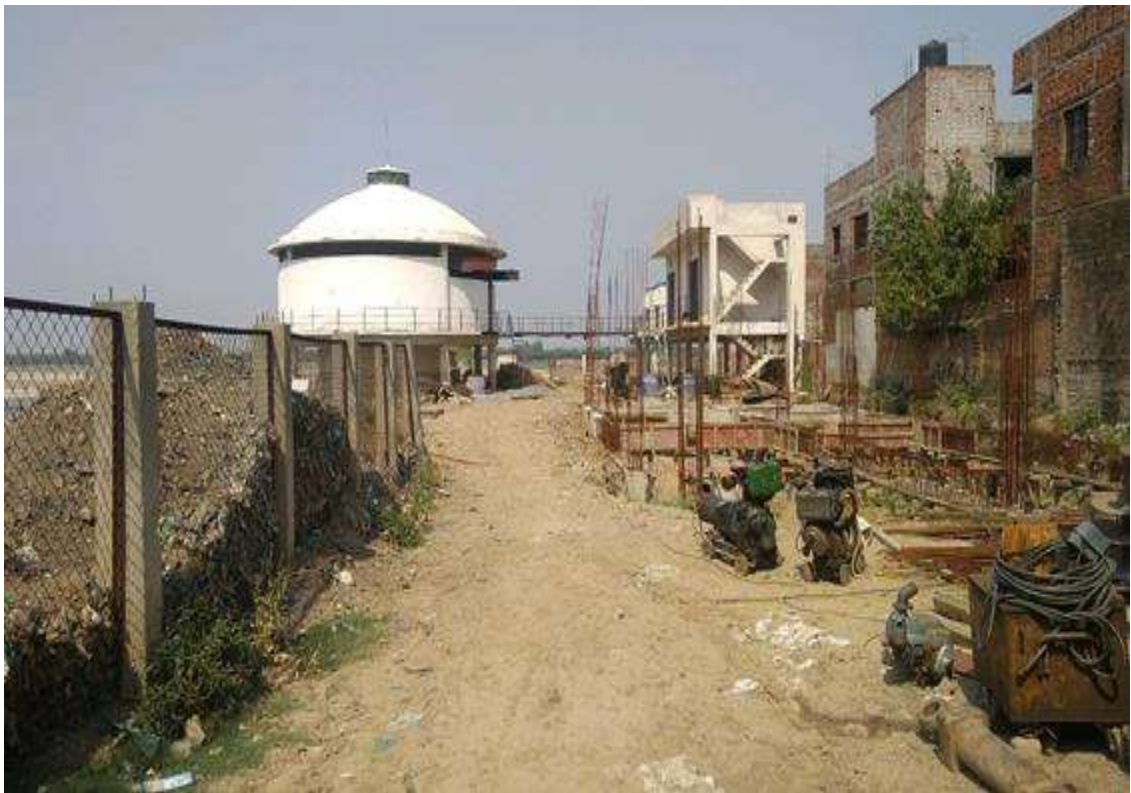
Main pumping station
