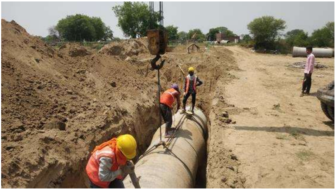
Treated effluent pipeline
