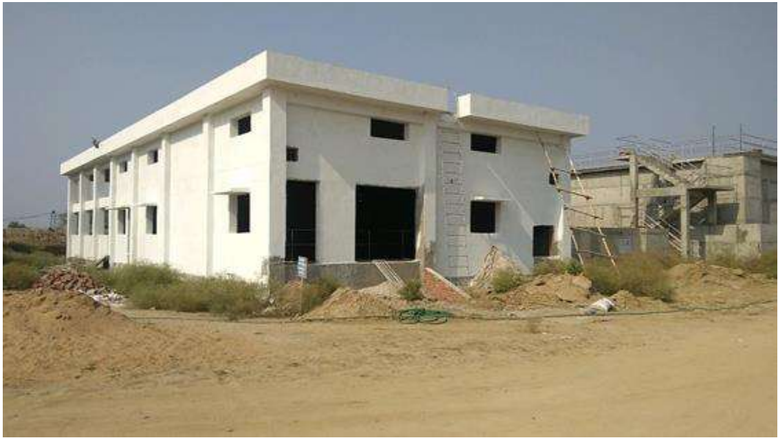
Treated water pump house
