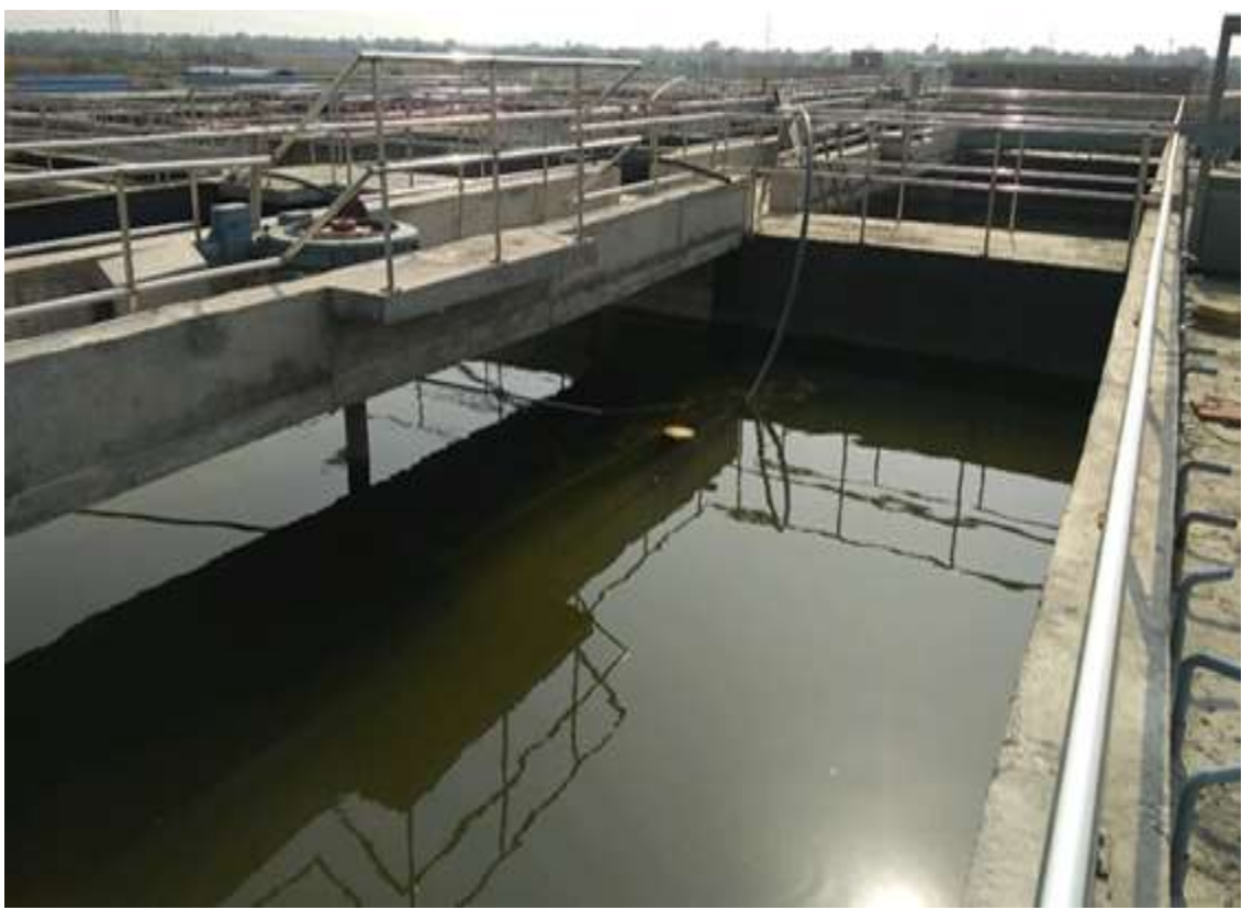
Grit removal basin
