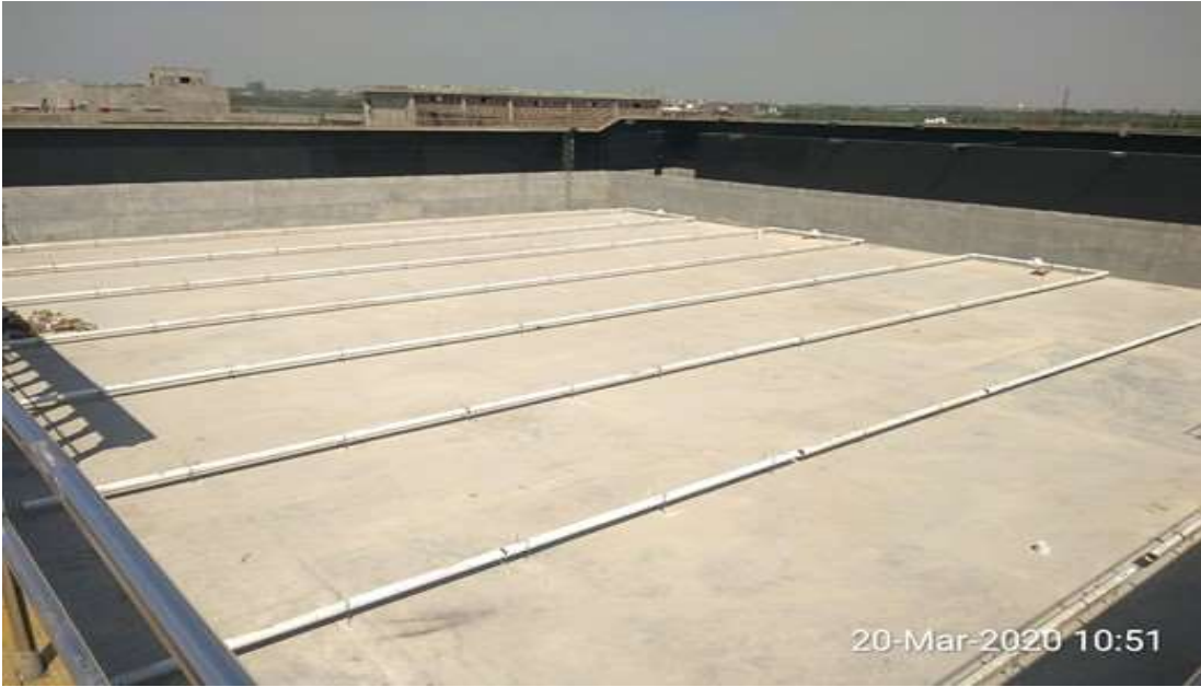
SBR -B3- Cable tray & Piping
