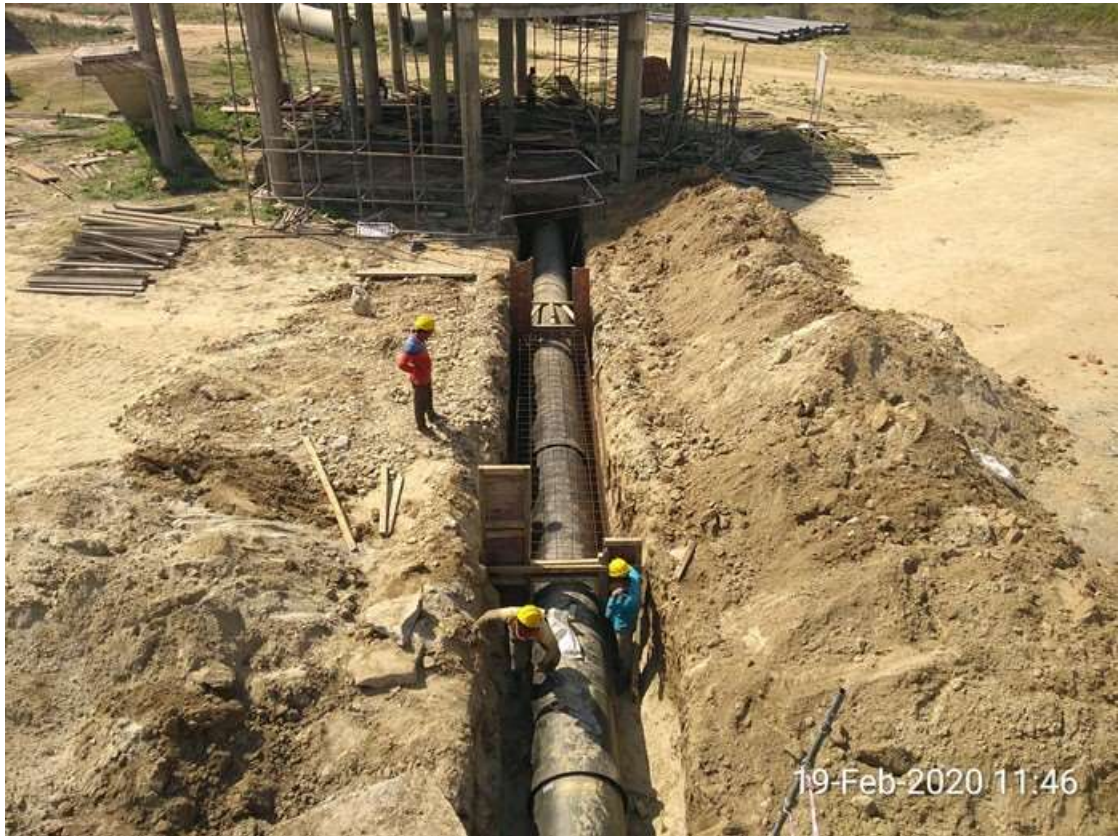
Treated effluent pipeline
