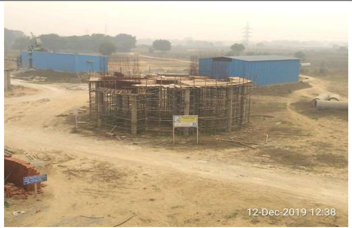
Over Head Tank (OHT)
