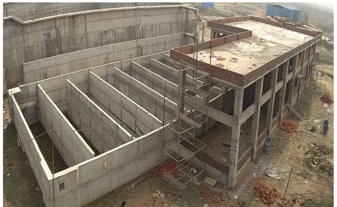
CCT – Treated water pump house
