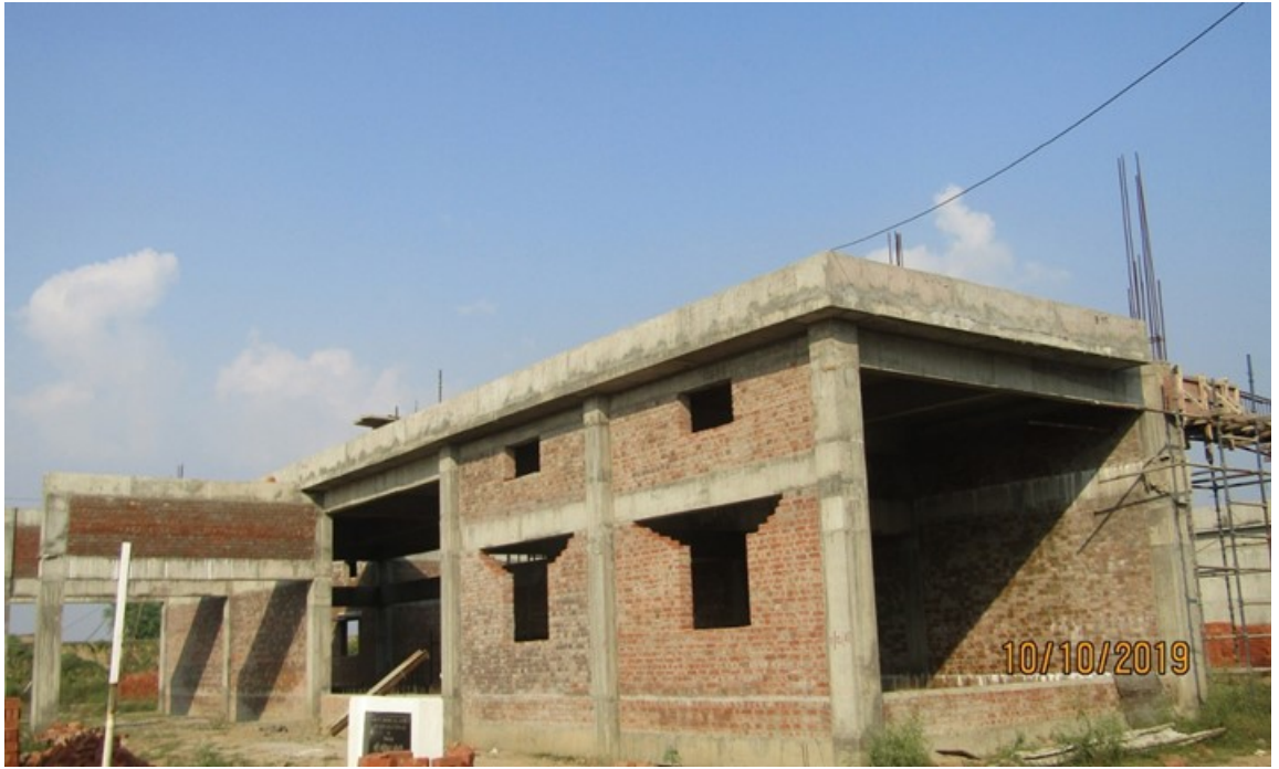
Air Blower & MCC Building
