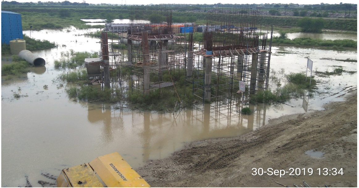
Over Head Tank (OHT)
