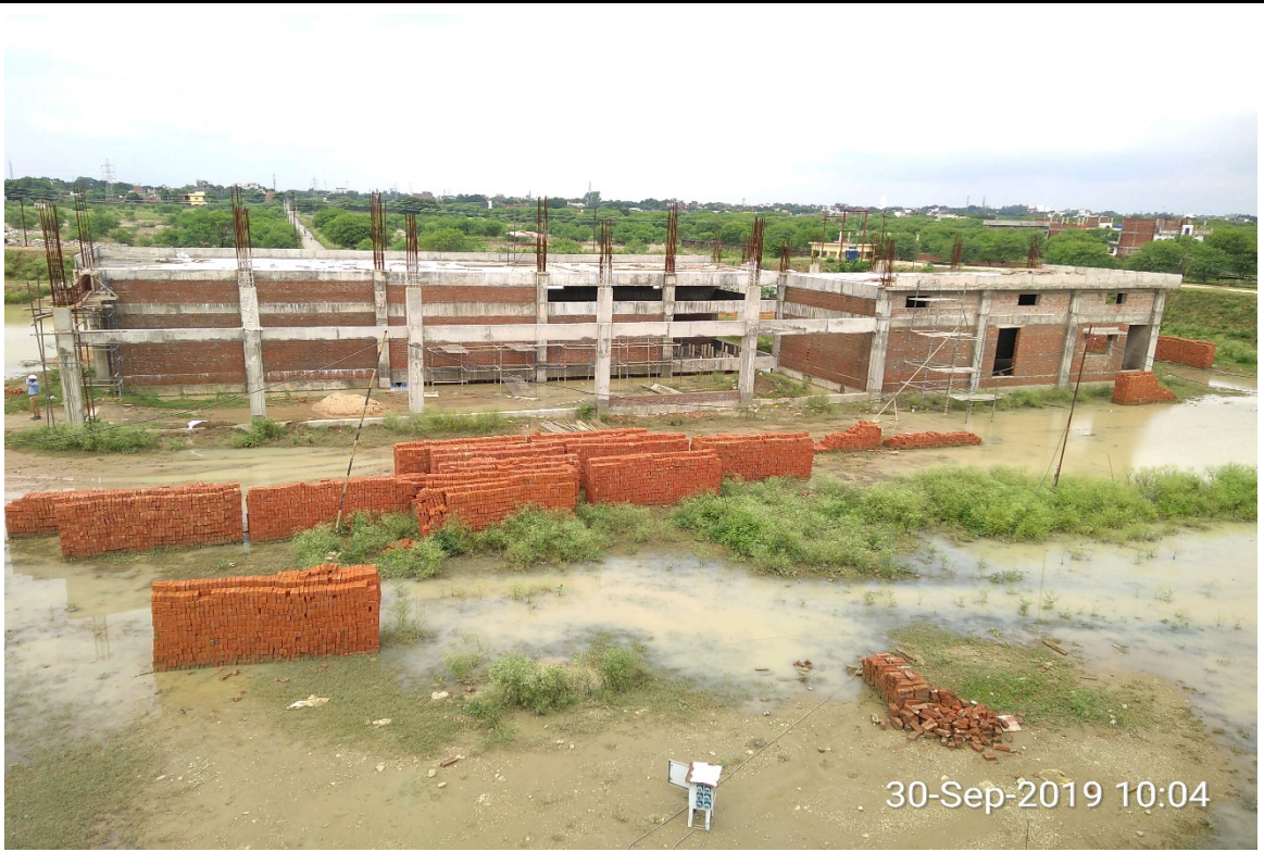
SBR air blower room, HT room, MCC room, Transformer Yard & DG set area
