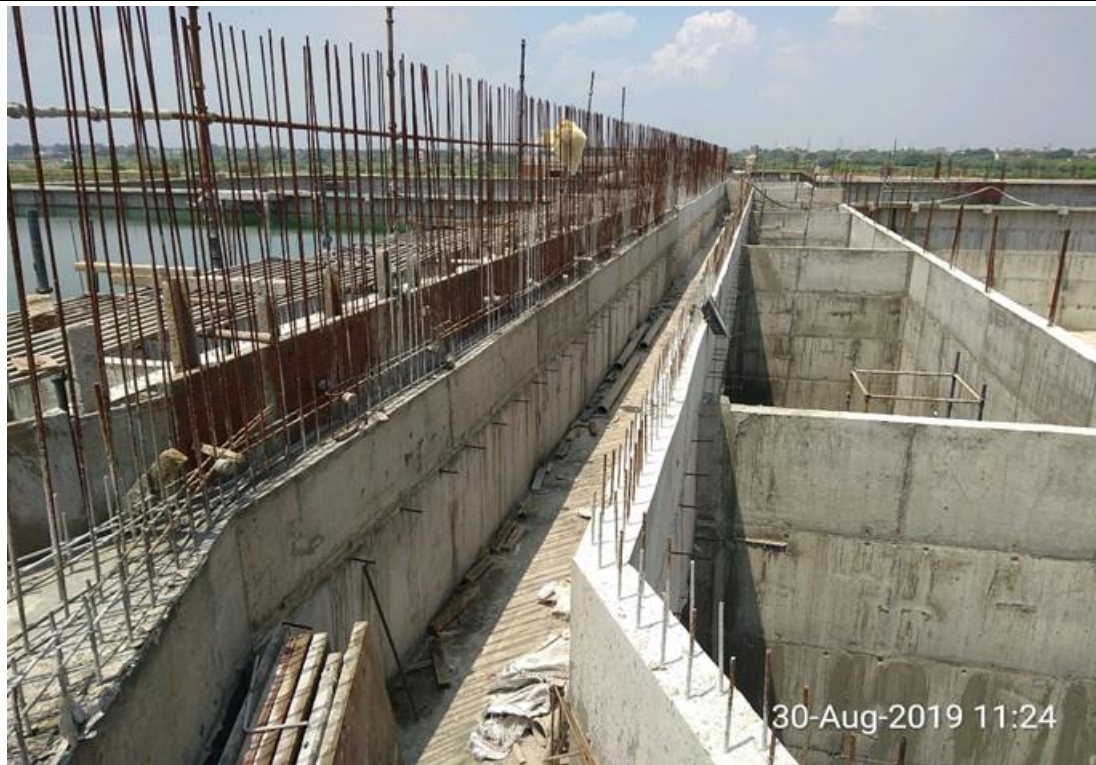
SBR Inlet channel
