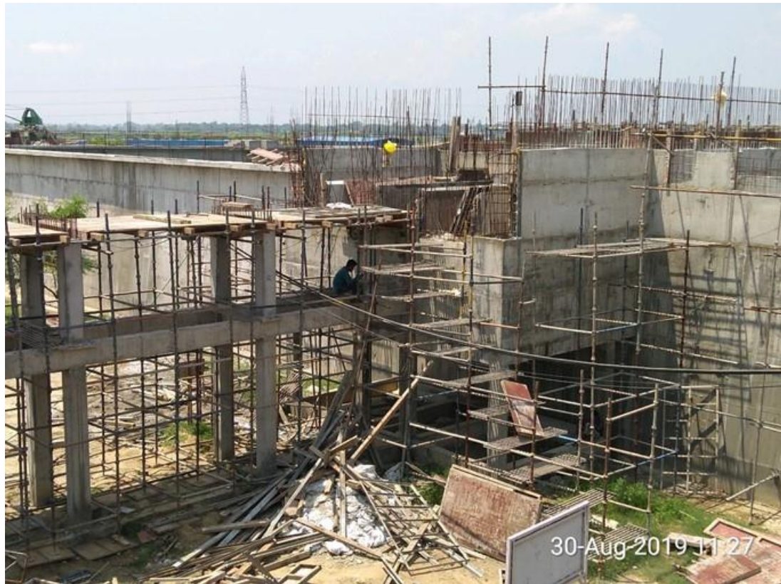
Parshall flume to SBR distribution chamber
