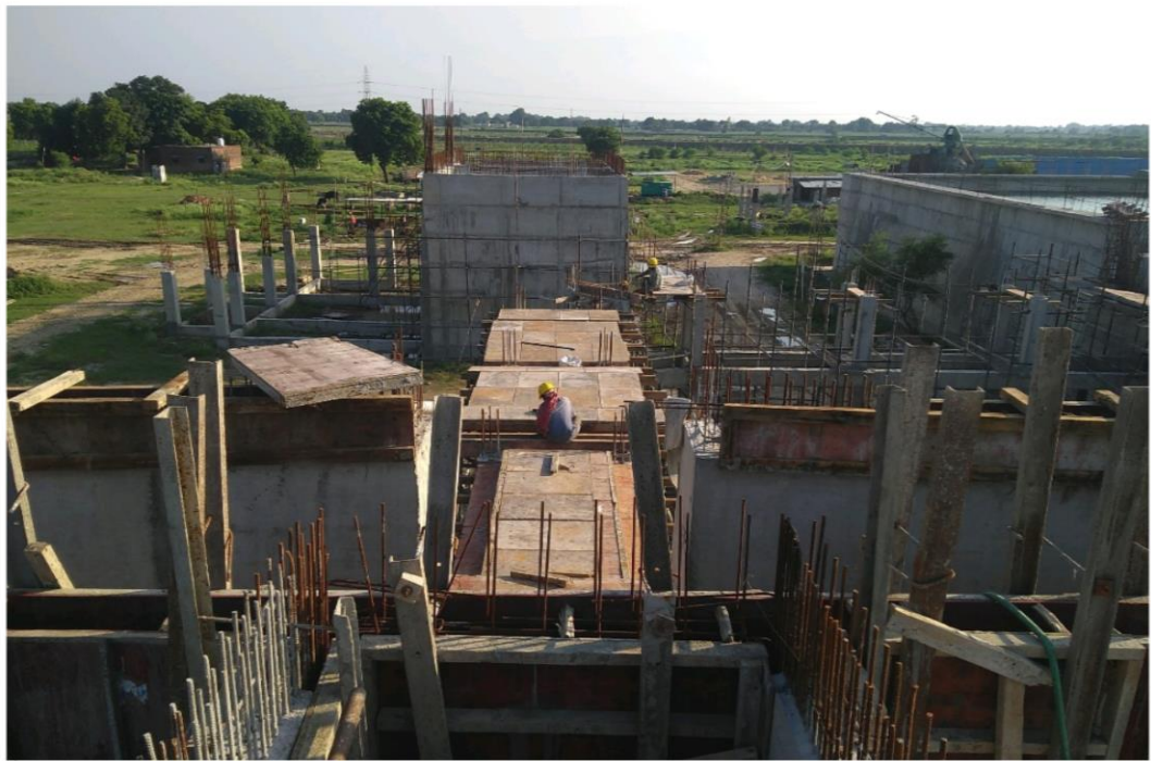
Grit chamber to Parshall flume to SBR distribution chamber
