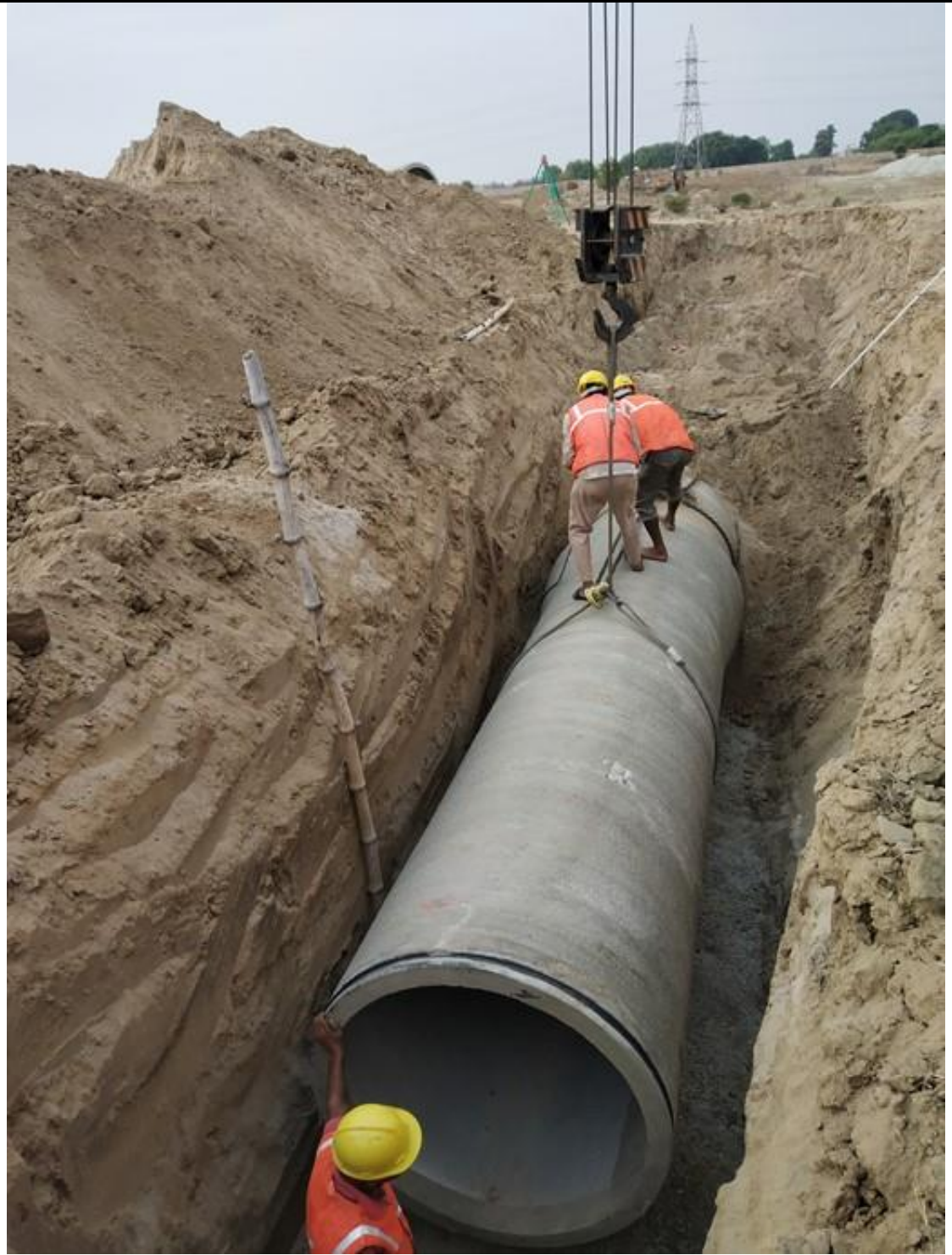
Treated water effluent line
