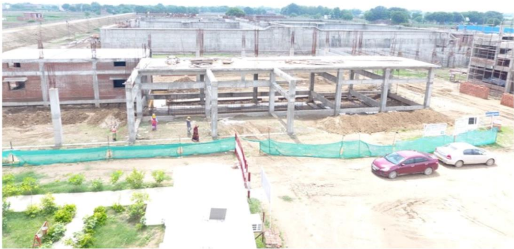
SBR air blower room, HT room, MCC room, Transformer Yard & DG set area
