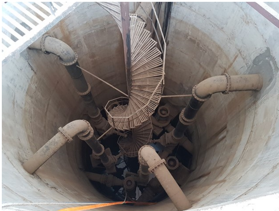
Existing collection well
